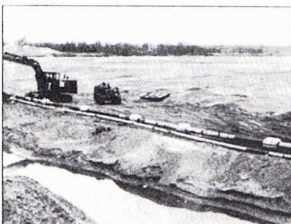
Fig. 2. Bolt-on concrete weights, which weighed 830 lb each, were not sufficient to prevent the pipeline from coming out.
