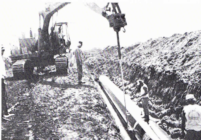
Cat 235 Backhoe used to install anchors on 42" Northern Border Pipeline in Iowa.
